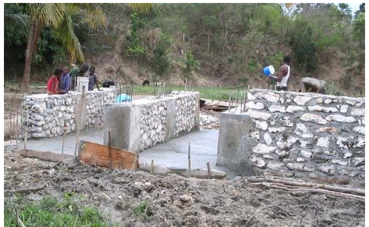
The Million Pennies Bridge foundations, begun with the pennies from St. Margaret's
