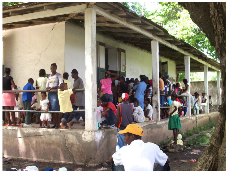
This picture of the clinic shows a beam in danger of collapsing on top of a child waiting for care.
