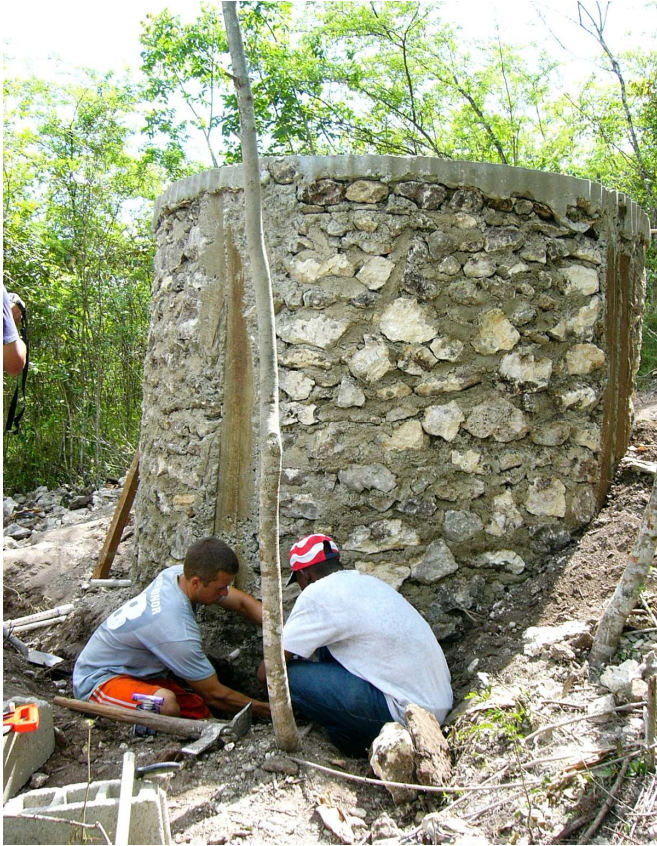
The new cistern on the hill above the school
